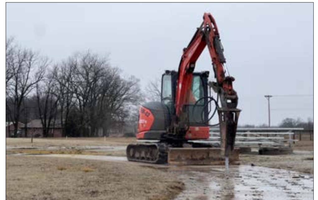
Removal of the sidewalk. Photo by Madalyn Richardson, Miami Tribe of Oklahoma (MTO).
